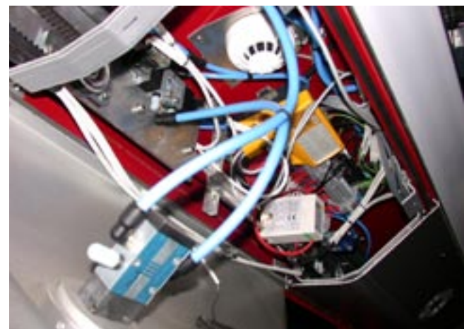
Remote I/O modules (yellow) in the roof compartments for door and compartment controls.
