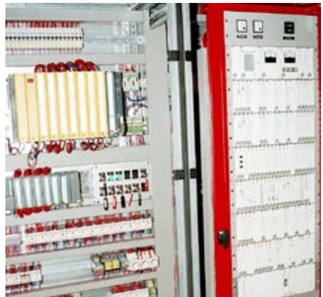
A view inside the control panel. Left, the fail safe PLC (yellow) and the Remote Supervision System rack on the right.
