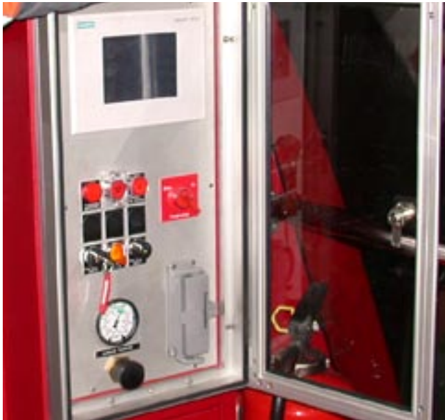
Downhill side emergency control station with touch panel and important controls and indications. This control station is normally locked..
