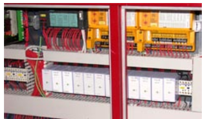
Control cabinet in upper drivers compartment with PSS I/O modules, S7 Profibus controller and common vehicle electric. Layout is clear and maintenance friendly.
